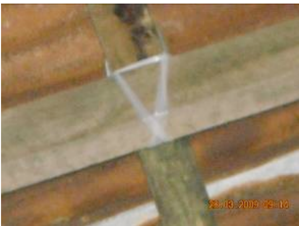
Purlin-rafter connection using fishing rope
