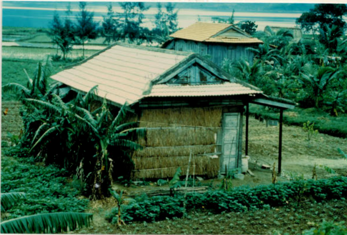
Contemporary 'transition' houses, weakened against typhoons by a mixture of materials and techniques
