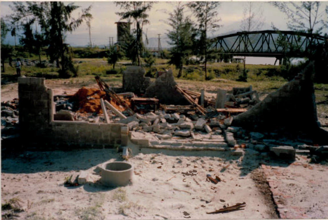
Cement block walled house destroyed in small typhoon - a total loss of investment.
