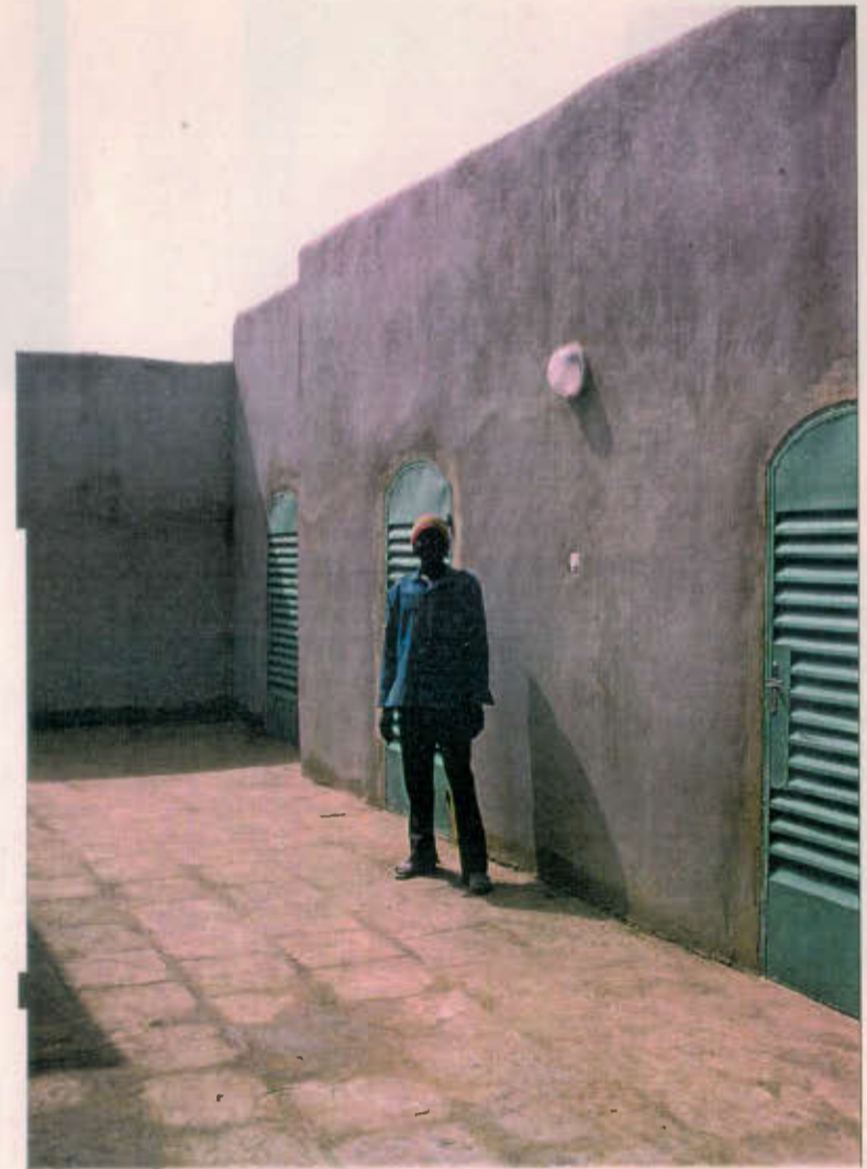
It is generally very important to evaluate the performance of a building during the first rainy season after its construction, in terms of water run-off, erasability, etc. In the case of the interior courtyard (shown above), we noted the mess created as the mud-plaster was washed off and deposited on the paving, and had the walls replastered in a ferro-cermit render.
